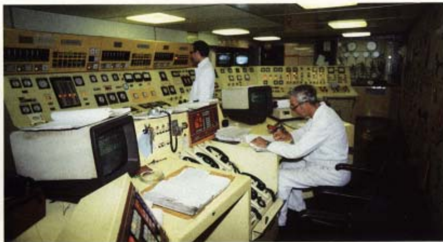
The boiler control room of the QE2 will be removed as part of the reengining to a diesel electric propulsion plant.
