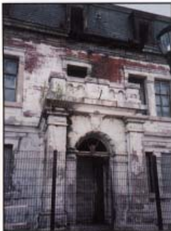
The 19th Century Operations Center of the old U.S. Lighthouse Service, on the U.S. National Register of Historic Places and a New York City landmark, will be rebuilt for the new museum.
